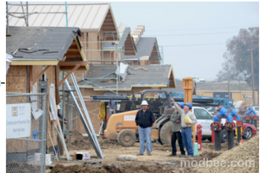
ELIAS FUNEZ/efunez@modbee.com Construction workers inspect a townhome site at Carver and 9th Street Wednesday afternoon. - The Modesto Bee - Elias Funez
